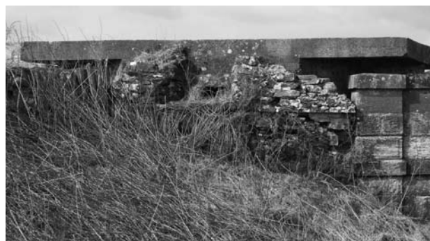
Illus 16 The pillbox at SEARCHLIGHT HILL (serial number South 5; Illus 15), showing the face camouflaged by stone at the west end of the railway bridge, overlooking the railway cutting. It is a Type 24 Bren Gun pillbox with an overhanging rectangular concrete roof which is clearly visible.
