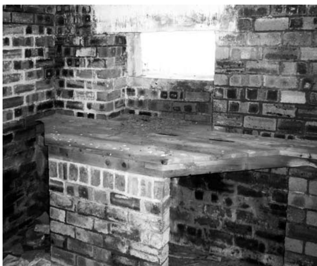
Illus 35 In the interior of the HANGAR VIEW pillbox the heavy timber shelves survive on which the Vickers machine guns would have been set.
